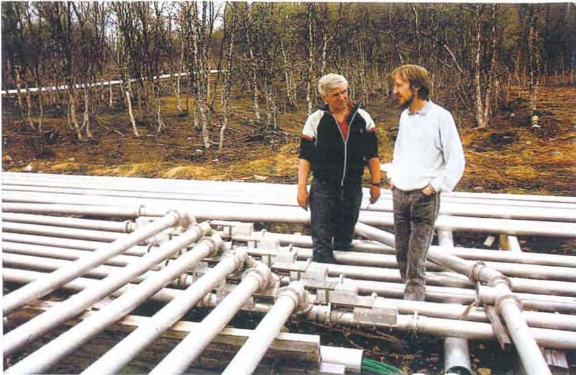
Fig. 12. The Heating Senior Scientist Dr. Michael Rietveld and Knut Helvig inspecting the antenna feed system of the Heating Facility at Ramfjordmoen.
